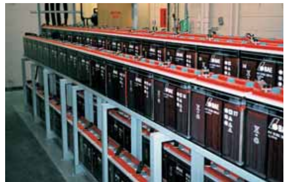
UPS application in USA 6 V 11 OGi 275
