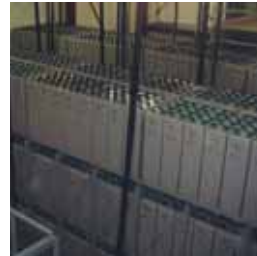
Colt Telecom in Amsterdam 24 OPzV 3000
